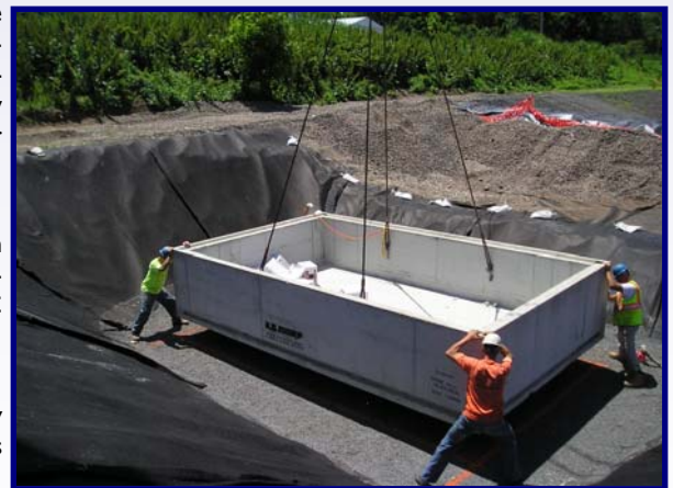
The Stone Hill Crew Stabilizes the Precast Structure for a Safe Placement
