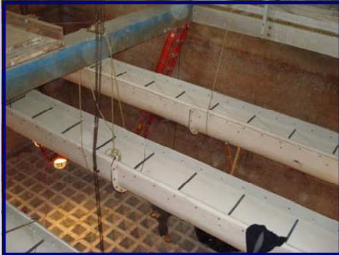
Fiberglass Collection Troughs for the New Filters
